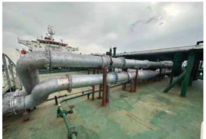
BWTS Piping on Deck
