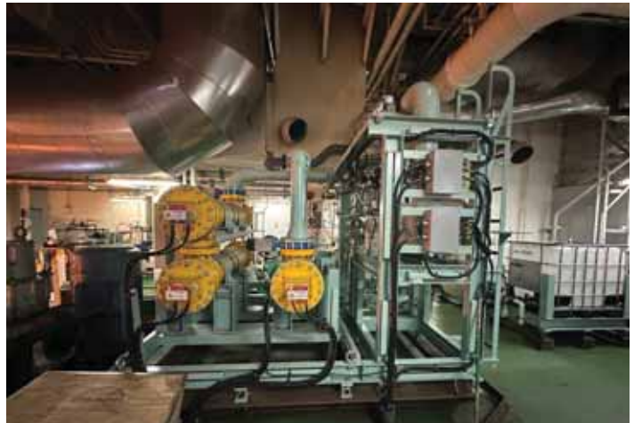
BWTS Electrolysis Unit
